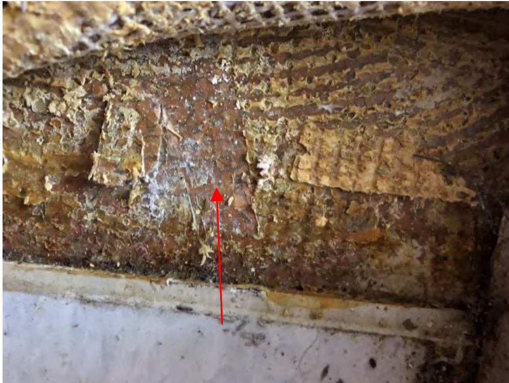
Photo 5: View of the asbestos-containing brown floor covering.
