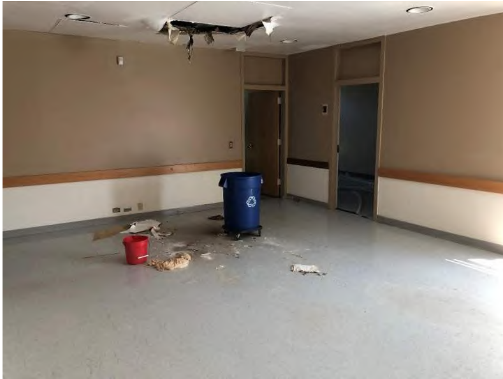
Photo 3: View of asbestos-containing drywall ceiling joint compound in room 217-20, where the ceiling has fallen down and created a disturbance.
