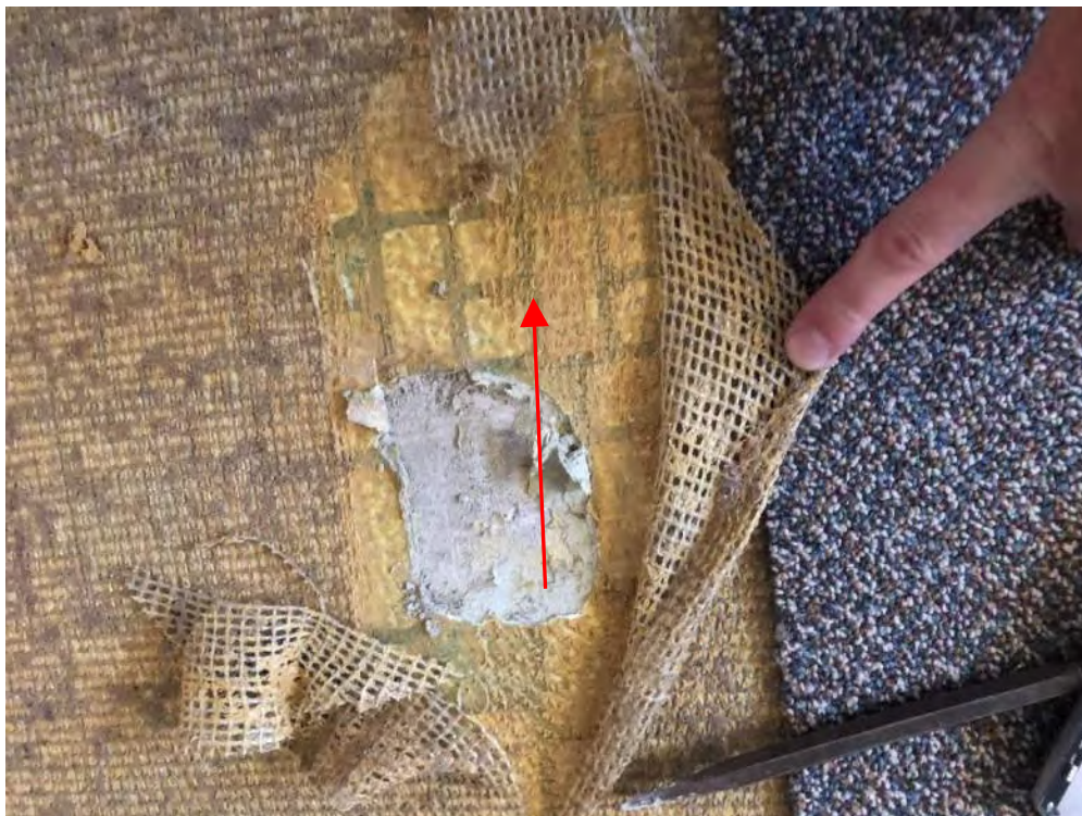
Photo 6: View of the asbestos-containing blue/tan floor covering.
