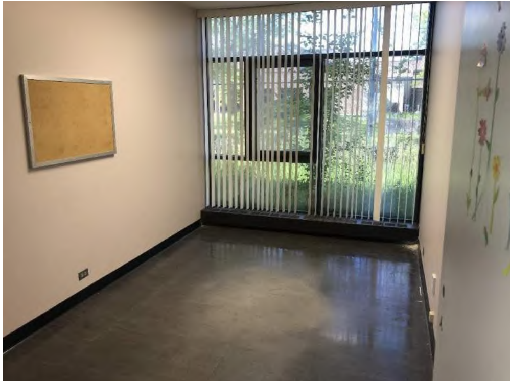
Photo 1: View of the asbestos-containing black 12"x12" floor tile. Associated black mastic is also asbestos-containing.
