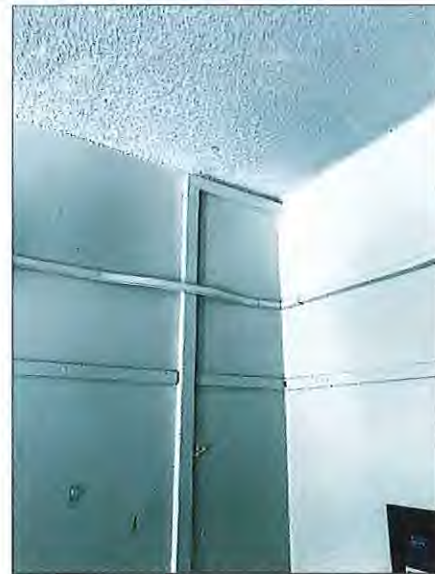
1 TYPICAL ELECTRICAL CONDUIT
