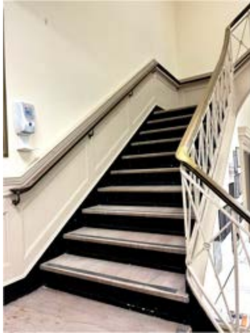
Photo 3: Tread and Riser Details
