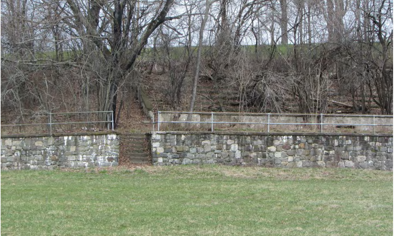
Photograph 22: Facing east from existing soccer field to close up of concrete grandstand and stone wall, now overgrown, built into the hillside.
