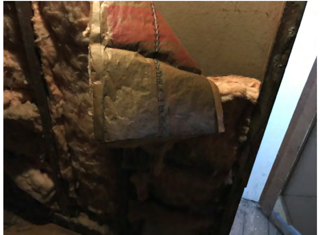
View of Second Floor Attic Area looking South at Access Door Wall
