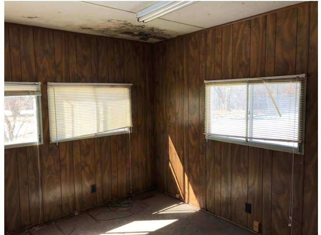
Interior Southwest Office with Apparent Mold Growth
