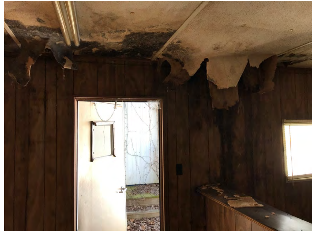
Interior Northwest Entry Room with Apparent Mold Growth
