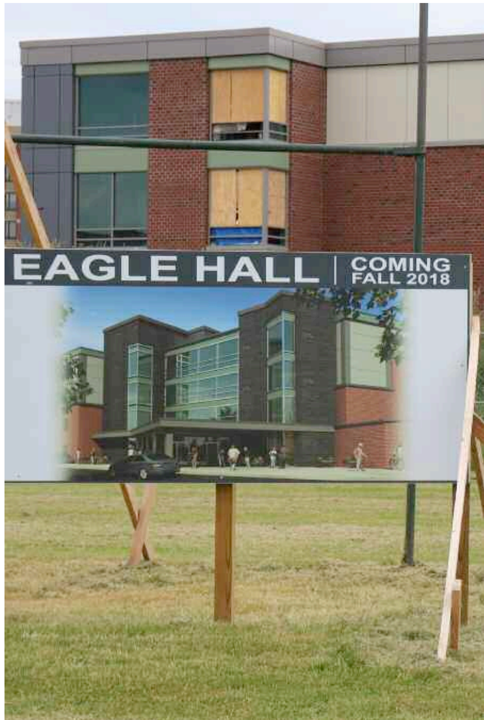
Dr. Gerrard Bushell, Rob Ryan, DASNY Director Construction/Western NY, and College President Dr. Heidi Macpherson toured the construction underway at the new residence hall in June 2018.
